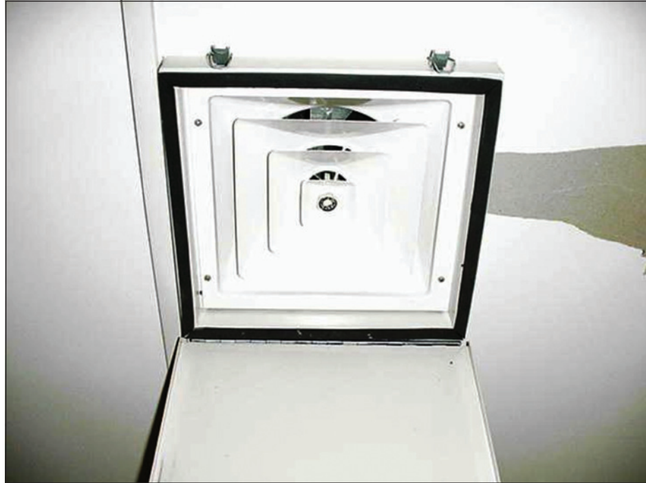
Figure 5-6: A hinged cover for sealing the supply vent of a safe room
